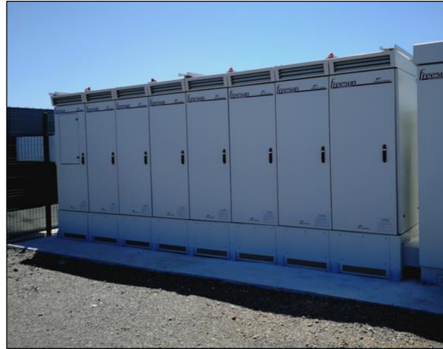
Typical centralised inverter
