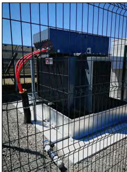
Plate 3-7. Typical outdoor transformer
