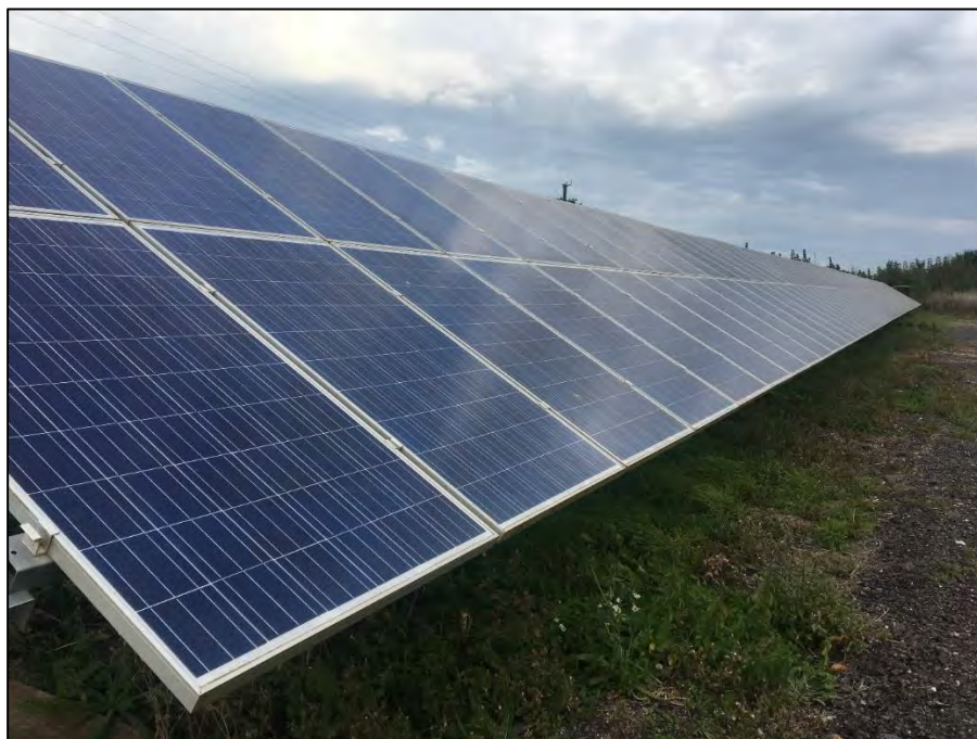
Plate 3-2. Solar panels with south facing configuration
