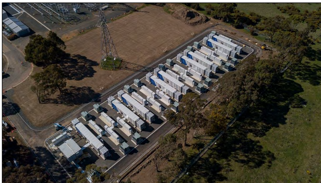
Plate 3-10. Typical battery storage compound configuration ( image reproduced courtesy of Fluence Energy ).
