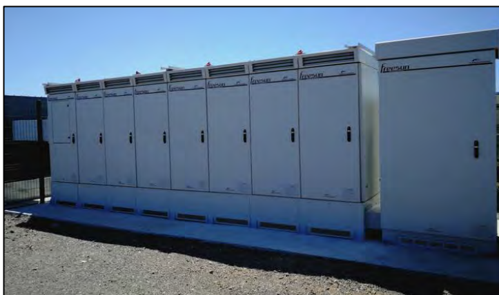
Plate 3-6. Typical outdoor centralised inverter
