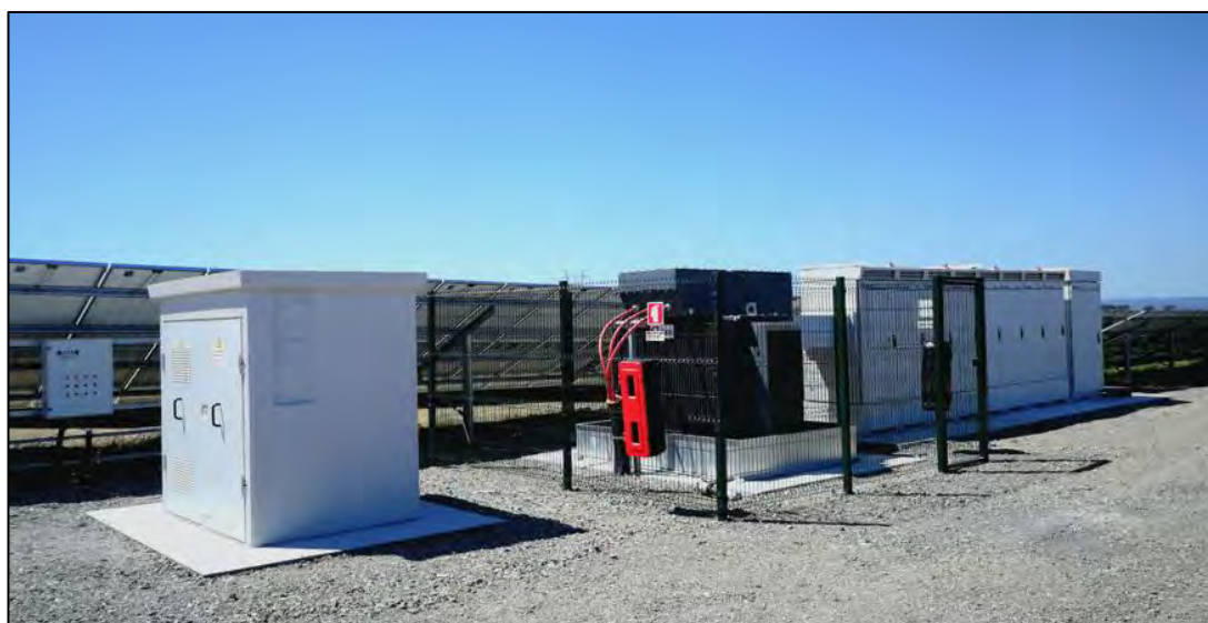
Plate 3-3. Outdoor solar station
