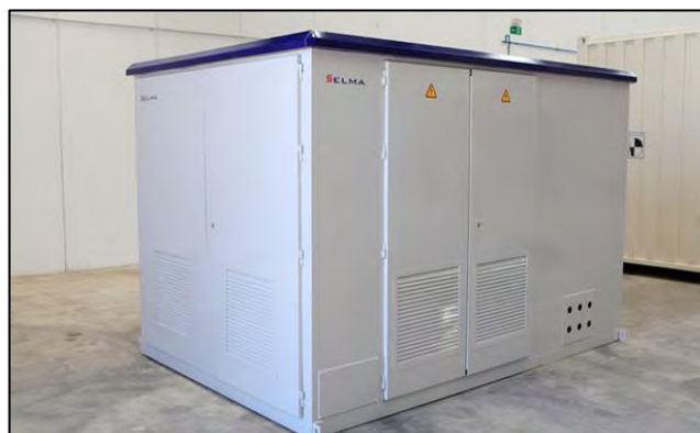
Plate 3-8. Typical transformer cabin (including switchgears) (indoor solar station) (Image reproduced courtesy of Selma)
