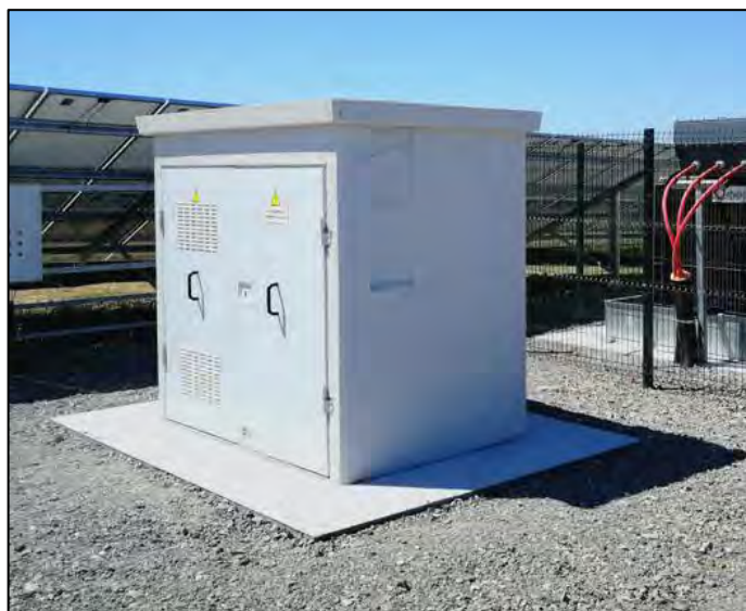
Plate 3-9. Cabin indoor switchgear used in the outdoor solar station solution.
